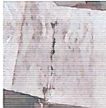
Photograph 4 ↑ Looking at mould growth on the surface of paper files, located in document binders.
