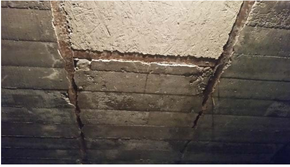
Photograph 1 ↑ Looking at concrete ceiling (and patch) located in former file storage room, in basement, where historic water intrusion events have occurred from.
