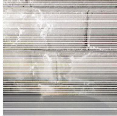
Photograph 2 ↑ Looking at concrete block wall located in the former file storage room, in basement, where mould growth concerns existed (sample MW-B1).
